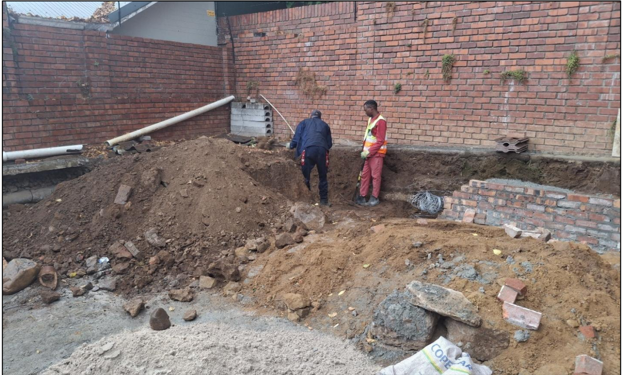
Working along the south-western edge of the property excavating a trench to build a retaining wall adjacent to the existing boundary wall. The new wall is partly already built. Upon going a deeper a grave was discovered directly beneath the worker in red.
