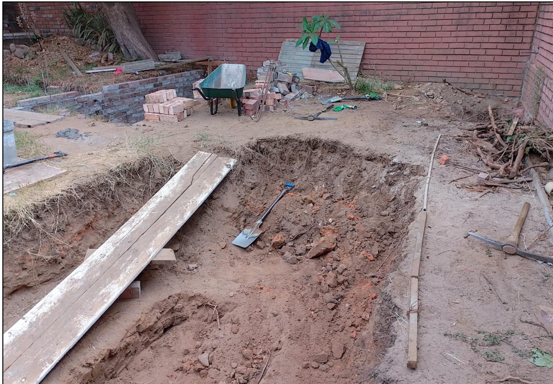
Excavation in the eastern corner of the property showing mostly fill but with some of the natural (and potentially sensitive) sand visible in the lower left part of the photograph.
