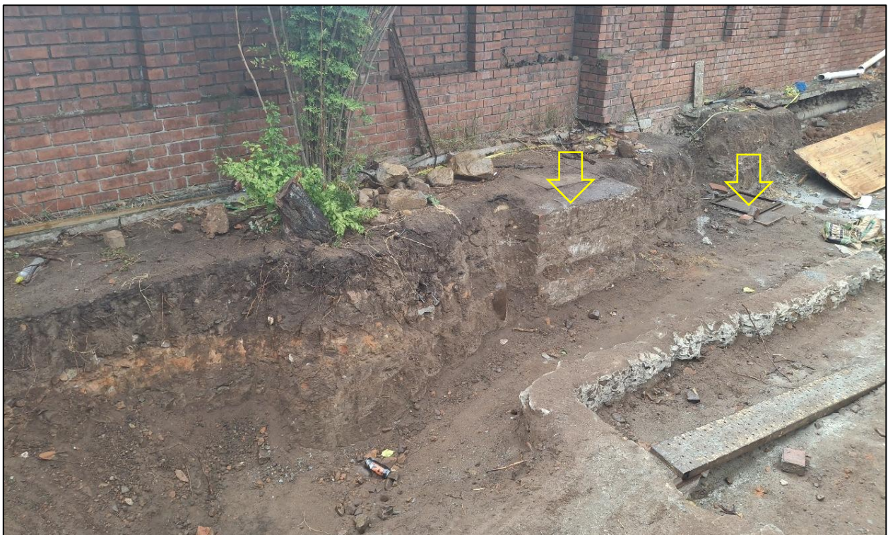
View of the section along the south-eastern boundary of the property showing existing manholes (arrowed; one has already had its upper part demolished) along a sewer line that runs parallel to the boundary wall.
