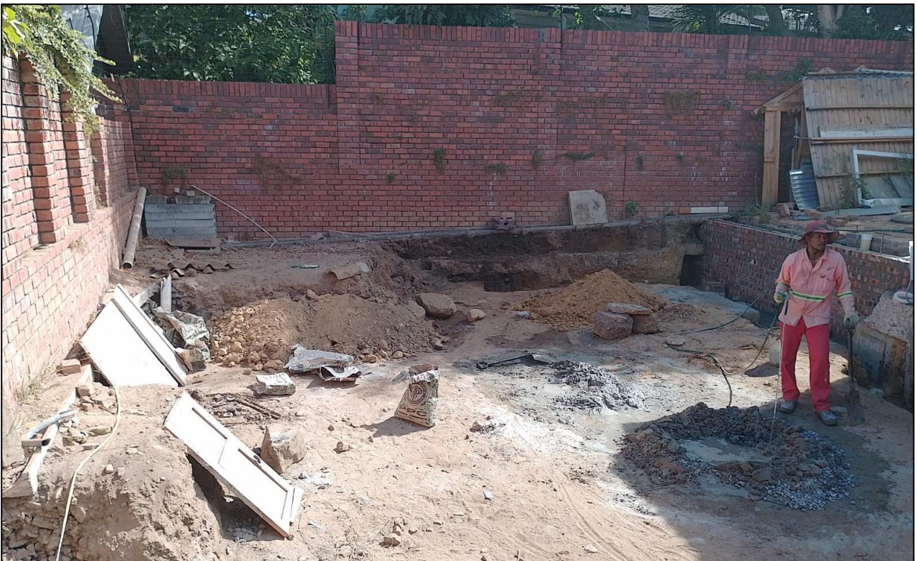
Excavation along the south-western edge of the property showing mostly fill but with some natural (and potentially sensitive) sand present at the base.
