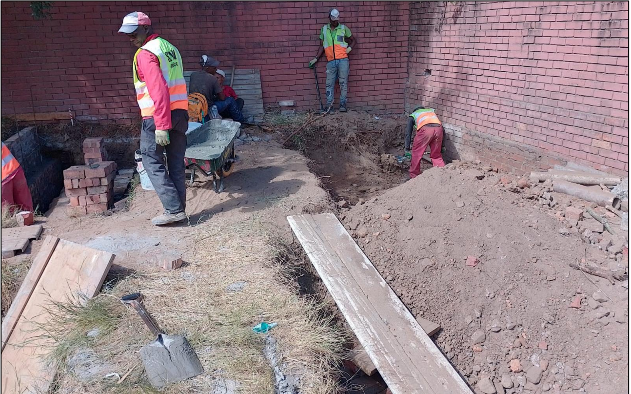
Continued excavation in the eastern corner of the property showing only fill.
