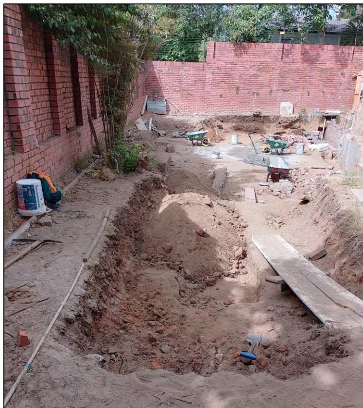
Excavation along the south-eastern edge of the property showing mostly fill but with the natural (and potentially sensitive) sand beneath the far end of the plank.
