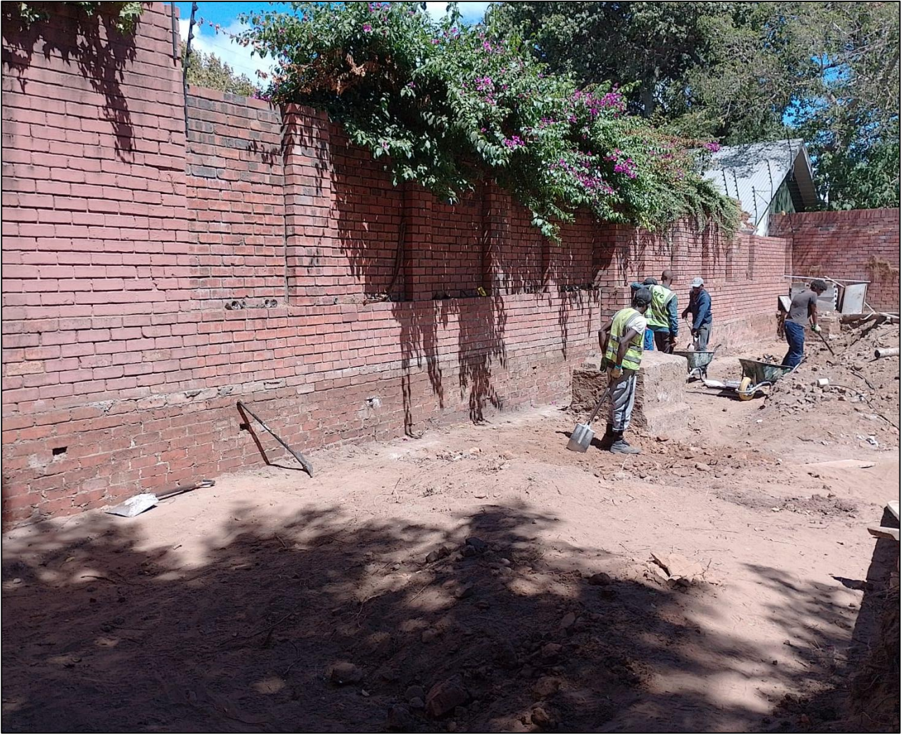
The entire strip along the south-eastern boundary wall has now been cleared.
