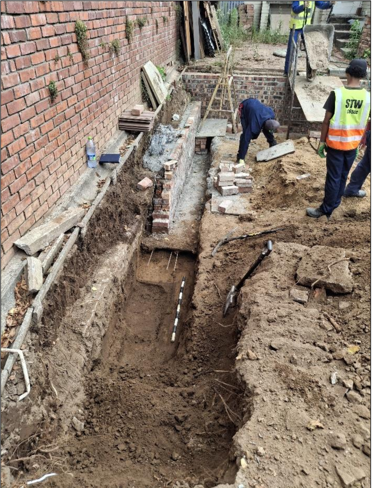
Looking northwest along the south-western boundary showing the location of the grave (immediately left of the black and white ranging rod in view) found on site on 13 February 2026. The grave is some 60 cm below the base of the foundation of the brick boundary wall and is some 9 m south-southwest of the location where the earlier human remains were discovered (out of picture towards the upper right).
