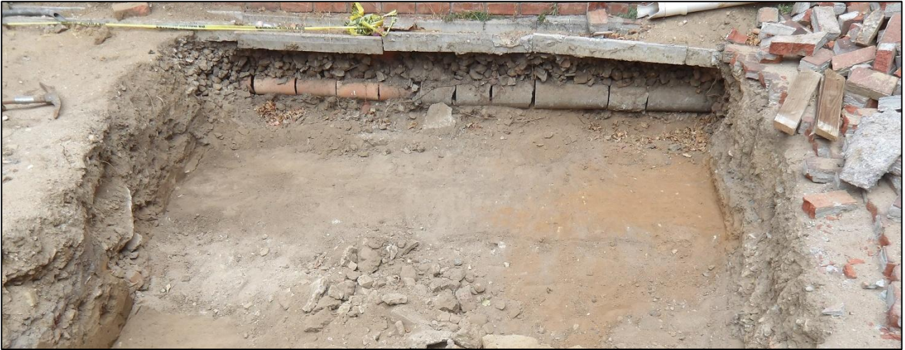
Figure 14: View towards the southeast showing the natural brown sand in the floor of the excavation to the left (NE) and the orange-brown fill to the right (SW). The French Drain is visible in the background in its gravel bed.
